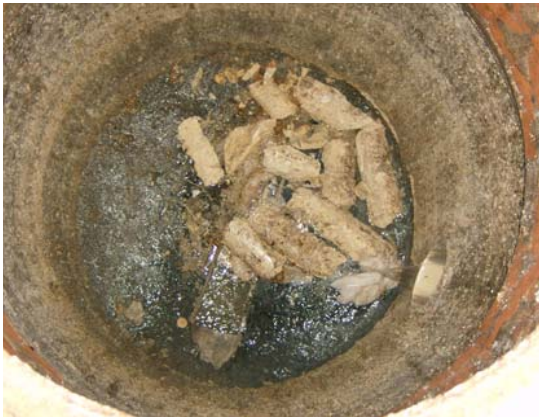
Grease from private lines accumulated in manhole.
